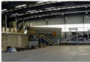
Organics Receiving Facility - ORF
