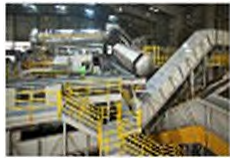
Material Recovery Facility - MRF
