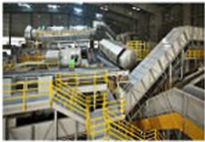
Material Recovery Facility - MRF
