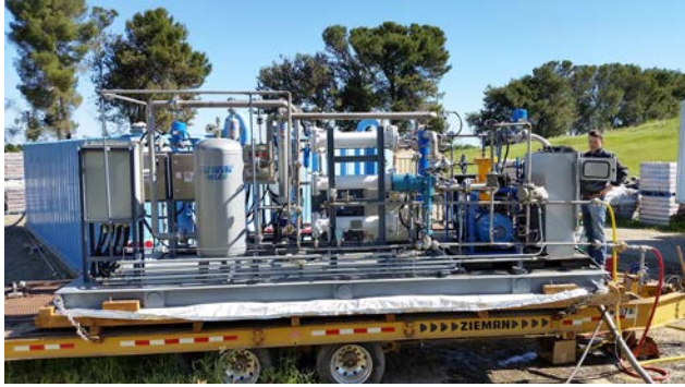
Figure 1-1: Helee upgrading unit on transportable trailer installed at UC Davis READ biogas facility.
