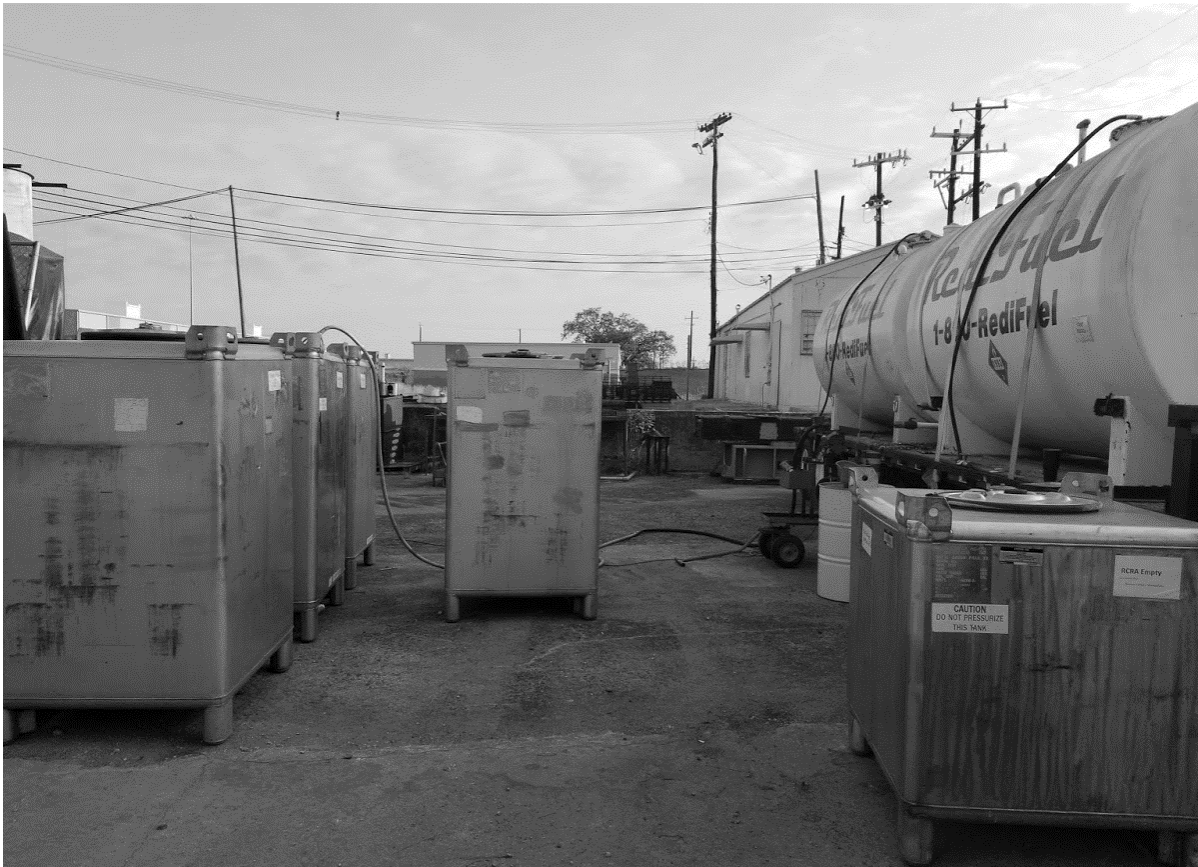
FIGURE 2. FUEL STORAGE TANKS
