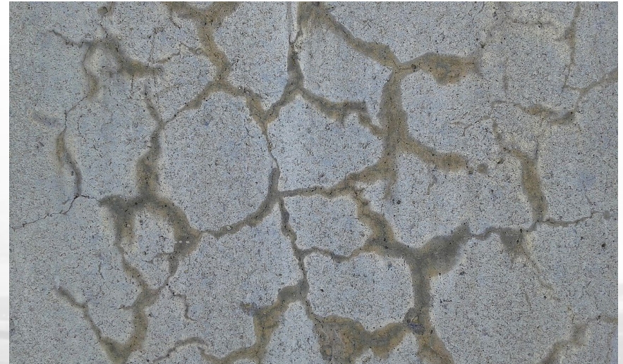
Pavement Deterioration due to Alkali-Silica Reaction (ASR), Caltrans Simi Valley
